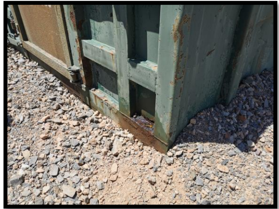
Photo 2: Evidence of a small hole in the waste skip at the substation, implying potential leakage of the skip.
