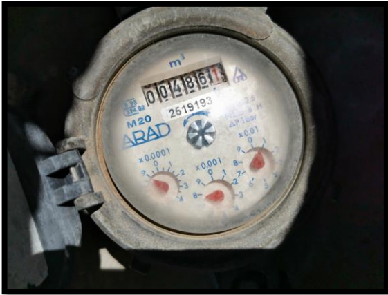
Photo 1: Water meter installed at the substation on site.
