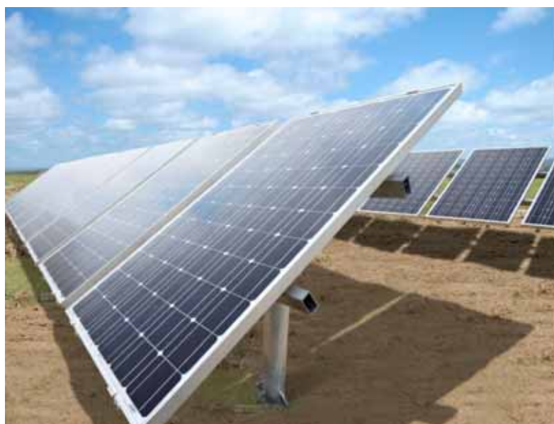
Figure 2.5: Photograph illustrating an array of PV panels.
